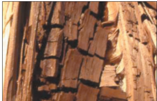
Photo 2d. Brown cubical rot. Brown rot fungi decay primarily the cellulose component of wood leaving the brown, brittle lignin as a residue.
