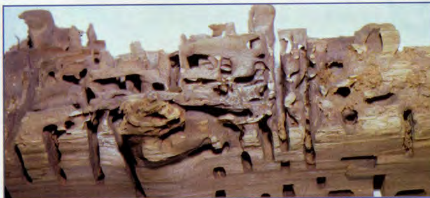
Figure 1. Carpenter ant excavation damage to a beam taken from a house.
