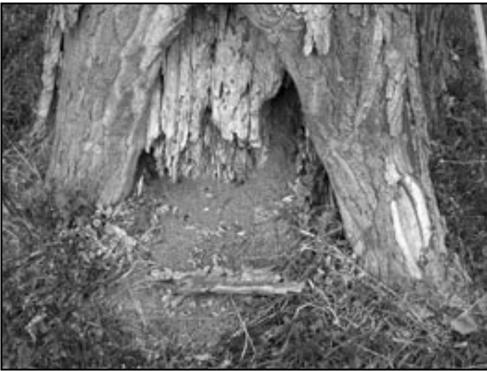
Photograph 4 - In most cases, decay was present but was not an immediate structural concern, as only 3% of the street trees sampled had more than 70% of the radius decayed. Decay incidence was high overall (58%) even in trees in the smaller diameter classes (53%).
