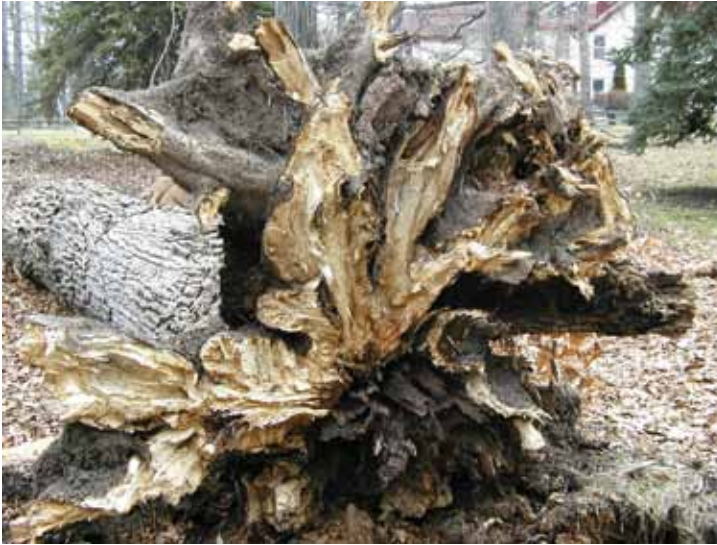
Figure 5. Sounding of roots near the base of a tree can be more difficult. However, roots with decay or have a poor connection to the soil may produce low, dull resonance on sounding, compared to normal roots with good soil connection. Interpretation of sounding results is more difficult, in general, with roots.
