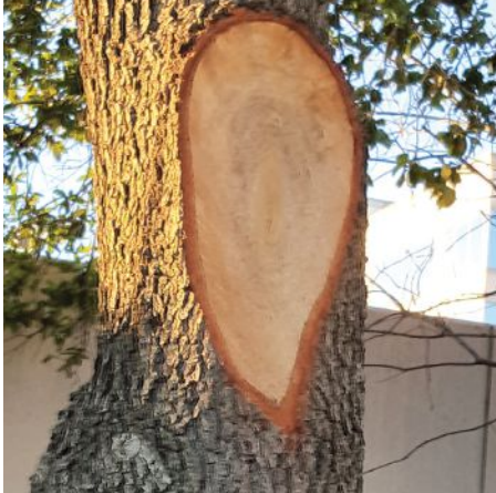
Photo 10: Large pruning wounds that expose heartwood and poor pruning practices, such as the flush cut shown here, can increase the likelihood of heart-rot infection. Photo courtesy of Chris Luley.
